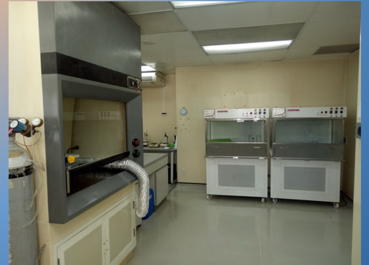
Hood and clean benches
